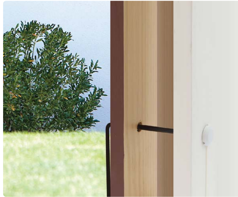
Figure 3. Round drop cable transitioning to 900-micron InvisiLight® cord inside the home.
